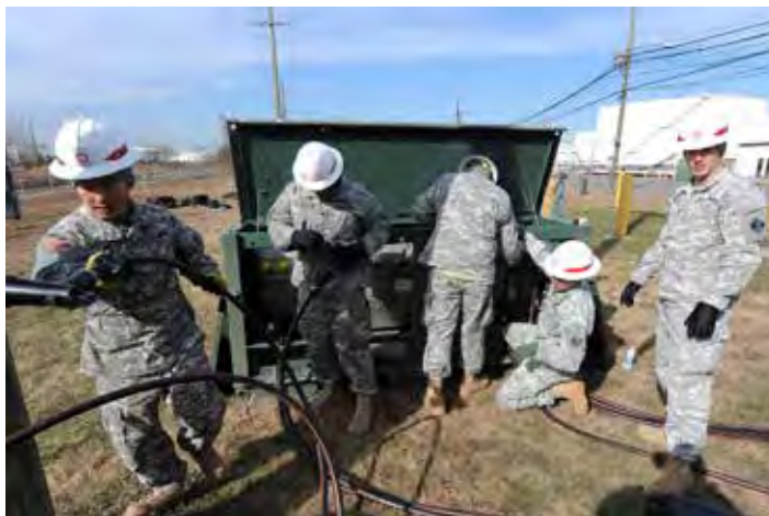
Soldiers from the 249th Engineer Battalion (Prime Power) install electrical generator equipment Nov. 6, 2012, at a Carteret, N.J., fuel depot that lost power during Hurricane Sandy. Power outages contributed to temporary gas shortages after the storm and getting fuel depots running was important to ending shortages. (DoD photo by EJ Hersom)
