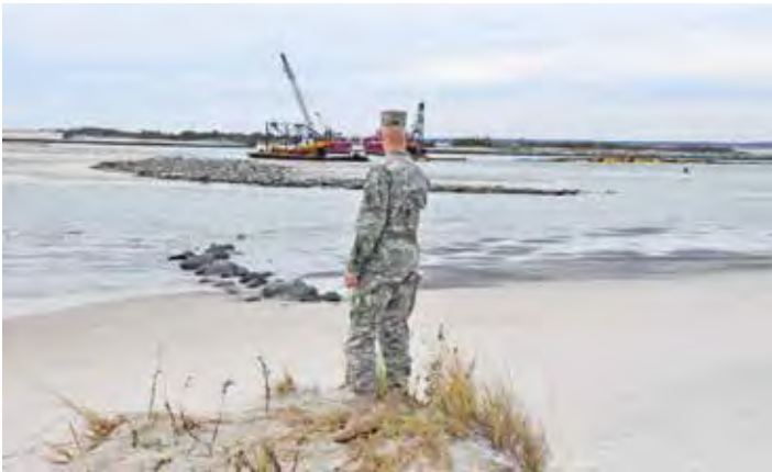
New York District Commander Col. Paul E. Owen stands on the edge of a dune and looks over a barrier island breach in Cupsogue County Park on Long Island Nov. 16, 2012, that was created by Hurricane Sandy. Crews are visible mobilizing to begin breach closure operations. (photo by Chris Gardner, New York District)
