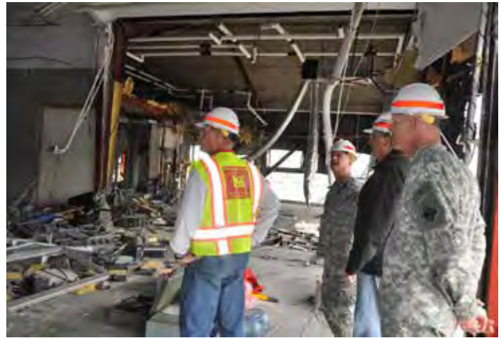
U.S. Army Corps of Engineers Deputy Commanding General Maj. Gen. Ken Cox surveys the severe damage at Caven Point on Nov. 2, 2012, with New York District leaders after Hurricane Sandy's storm surge devastated the facility. (photo by Chris Gardner, New York District)
